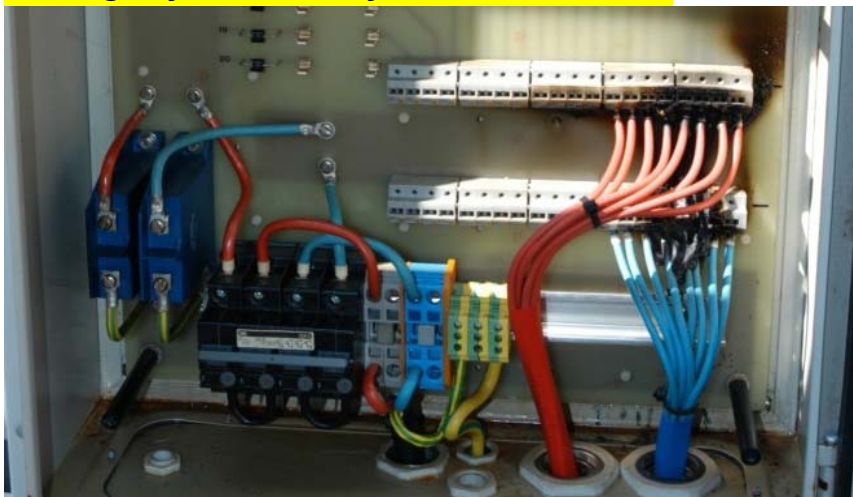
Damage caused by a smouldering fire, which occurred in the connector box of an 11 year old PV plant (15kW) in Burgdorf.
